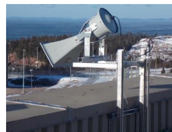
Community RMG-200AT at Point Lepreau
