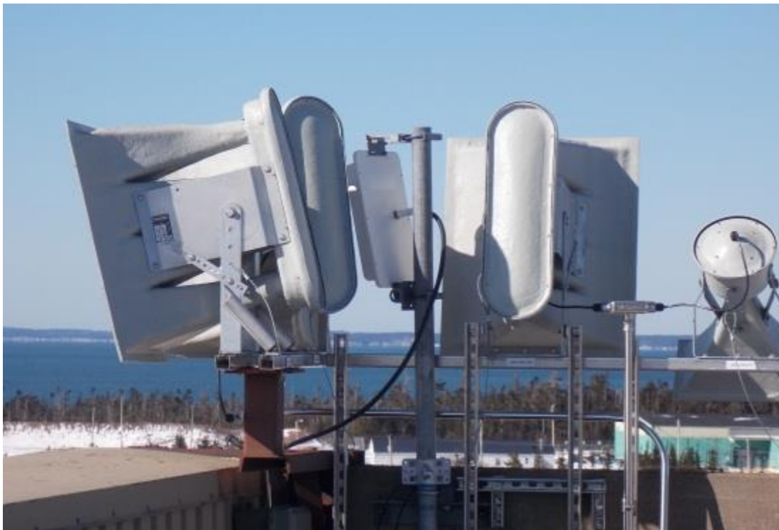
Community RSH-462 Loudspeakers at Point Lepreau Nuclear Generating Station in Halifax, Nova Scotia, Canada
